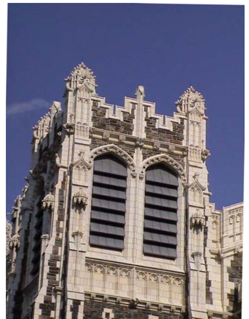
Shepard Hall, City College New York (1990's) 75,000 GRC elements with metakaolin and polymer addition
